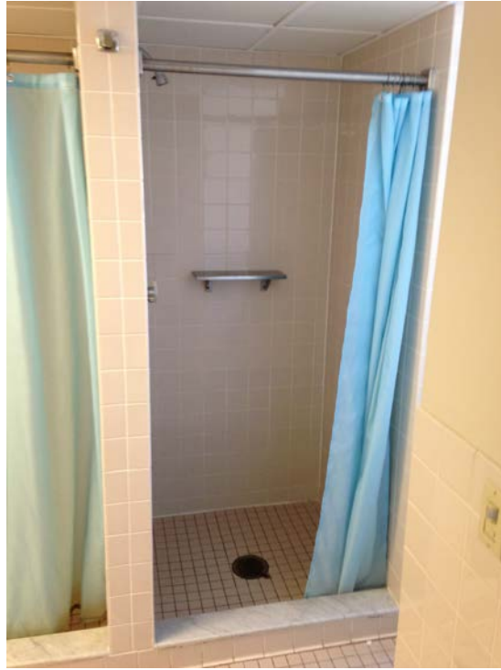
Northwest Ceramic Tile Shower - Leaks
