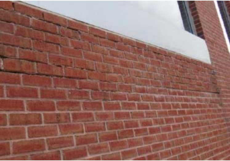
East Wall Façade Deterioration at Window Sill
